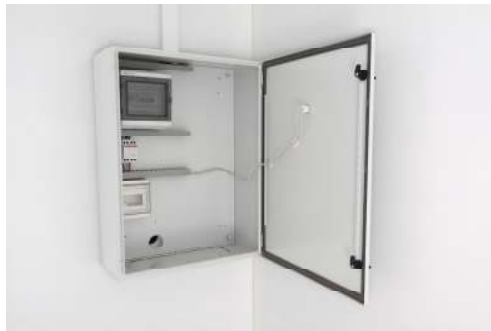
Interior view of shelter enclosure.
